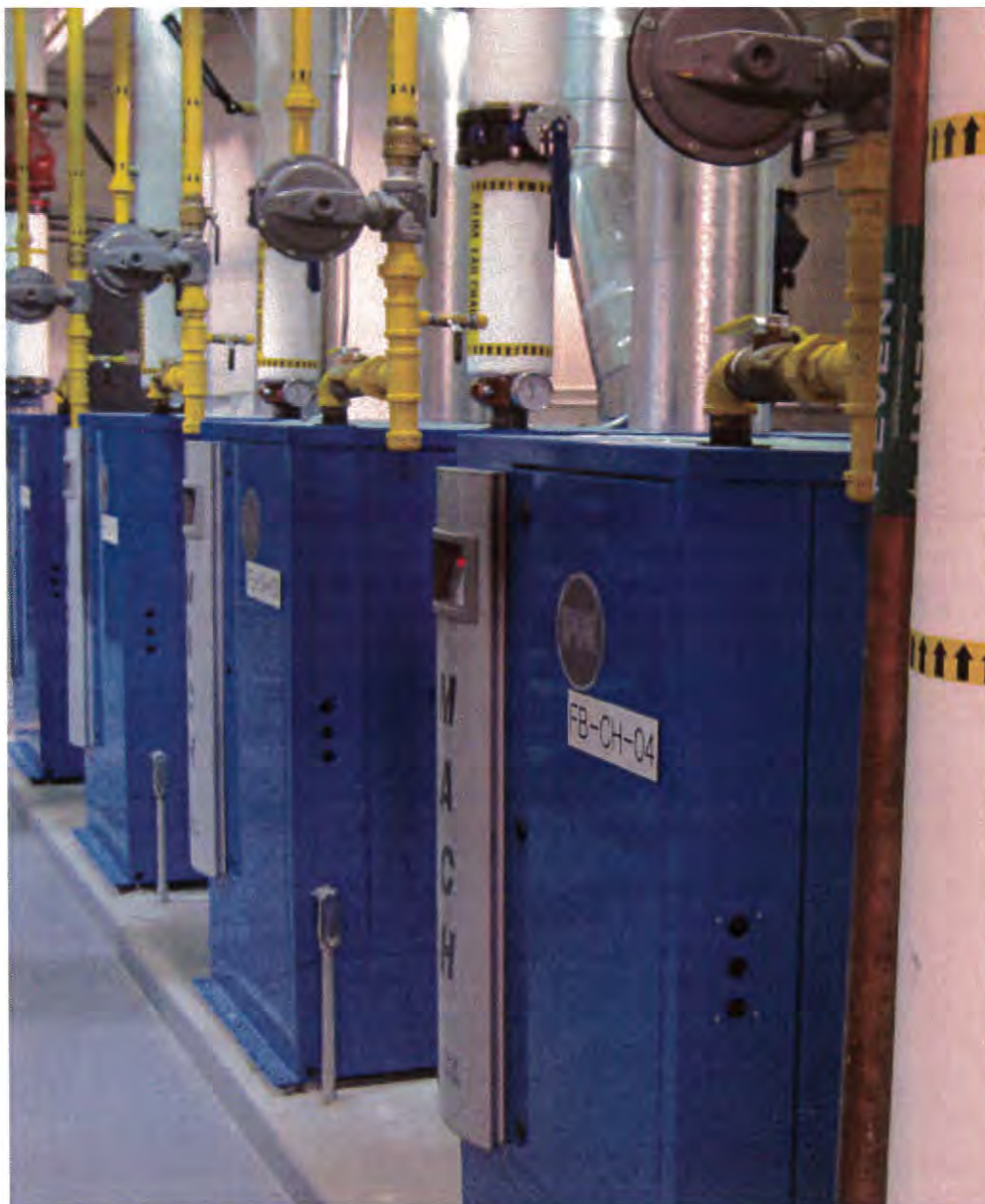
Patterson-Kelley, P-K MACH aluminum condensing boilers treated with TGWT’s tannin for more than three years, installed at a major hospital.
